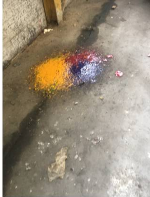
The only instance of an ink spill over a joint. Has not penetrated the joint.
