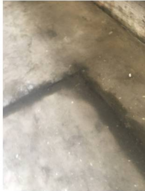
Worst-case examples of concrete pad joints
