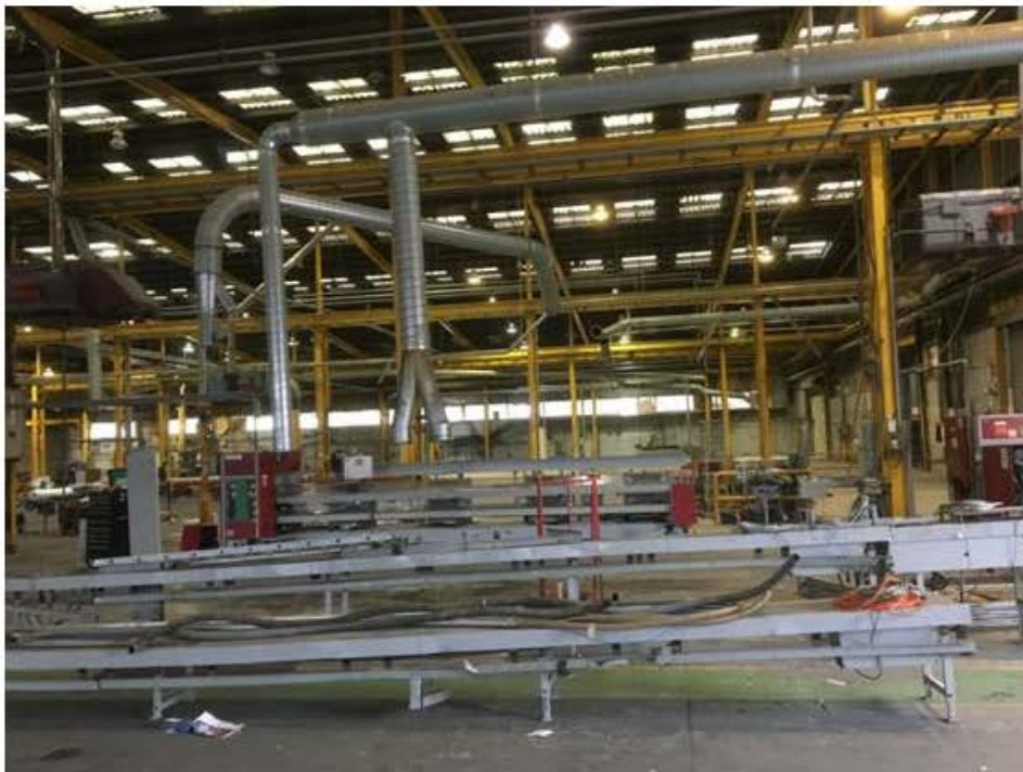
Photo 8 Ductwork (for paper trimmings) left in place, plus conveyors in the foreground prior to removal.
