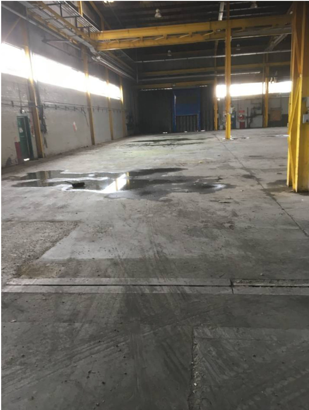
Overview of inside of factory eastern end. Note that the puddle is rainwater from damaged roof
