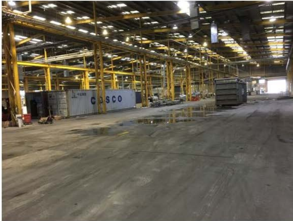
Photo 7 Main area, showing ingress of rain water through flues (the square tubes through the roof)
